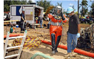
Greg West of Sea Engineering, who dived through 600 feet of sewer pipe to examine it for leaks, calls his job "adventurous" and "fun."
